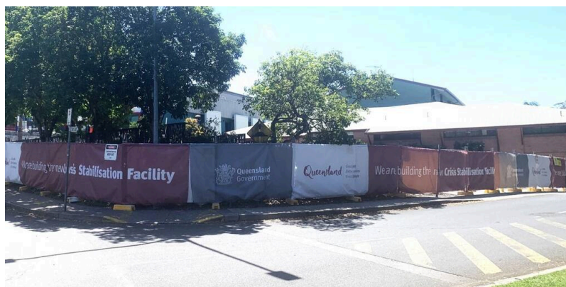
Preparation of the TPCH site is occurring ready for the delivery of the modular building in May.
